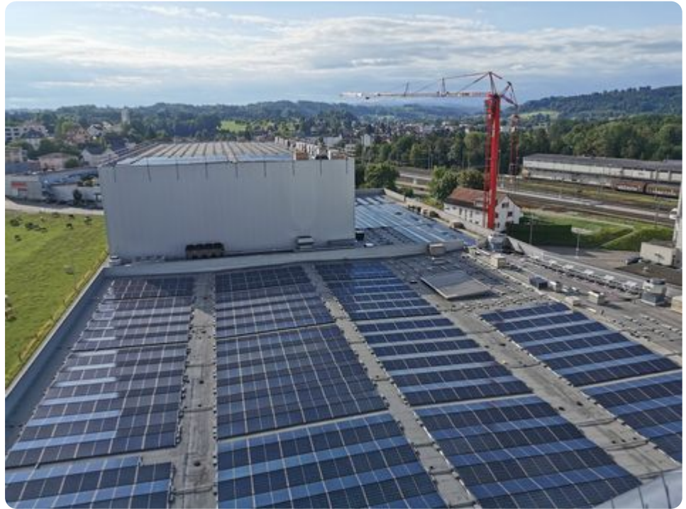
Photovoltaic system during the final phase of installation at the Sulgen site
